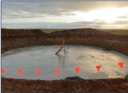
Stage 3. Foundation for Wind Turbine Generator Install Electrical Conduit and Blinding Concrete
