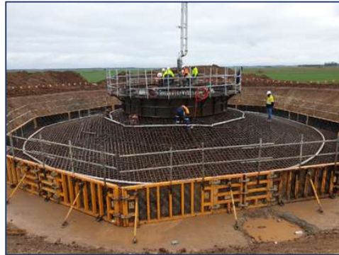
Stage 4. Foundation for Wind Turbine Generator Install Steel Work and Concrete Form Work
